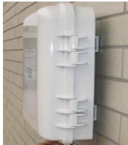
Mounted on the building (wall)
